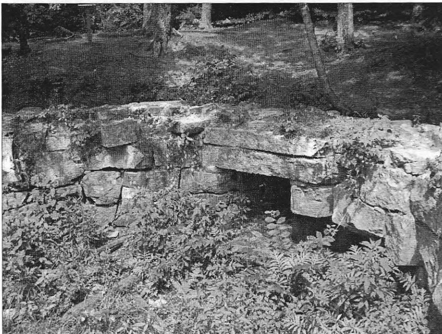
This circular pattern of stone is the foundation of the old "round mill" of the Oriental Powder Company in Gorham, Maine. Water from the nearby Presumpscot River drove two upright wheels which ground gunpowder components several inches thick. The trail in the background—now spotted with mature trees—is the towpath of the Cumberland and Oxford Canal, now part of the Presumpscot Regional Land Trust.
