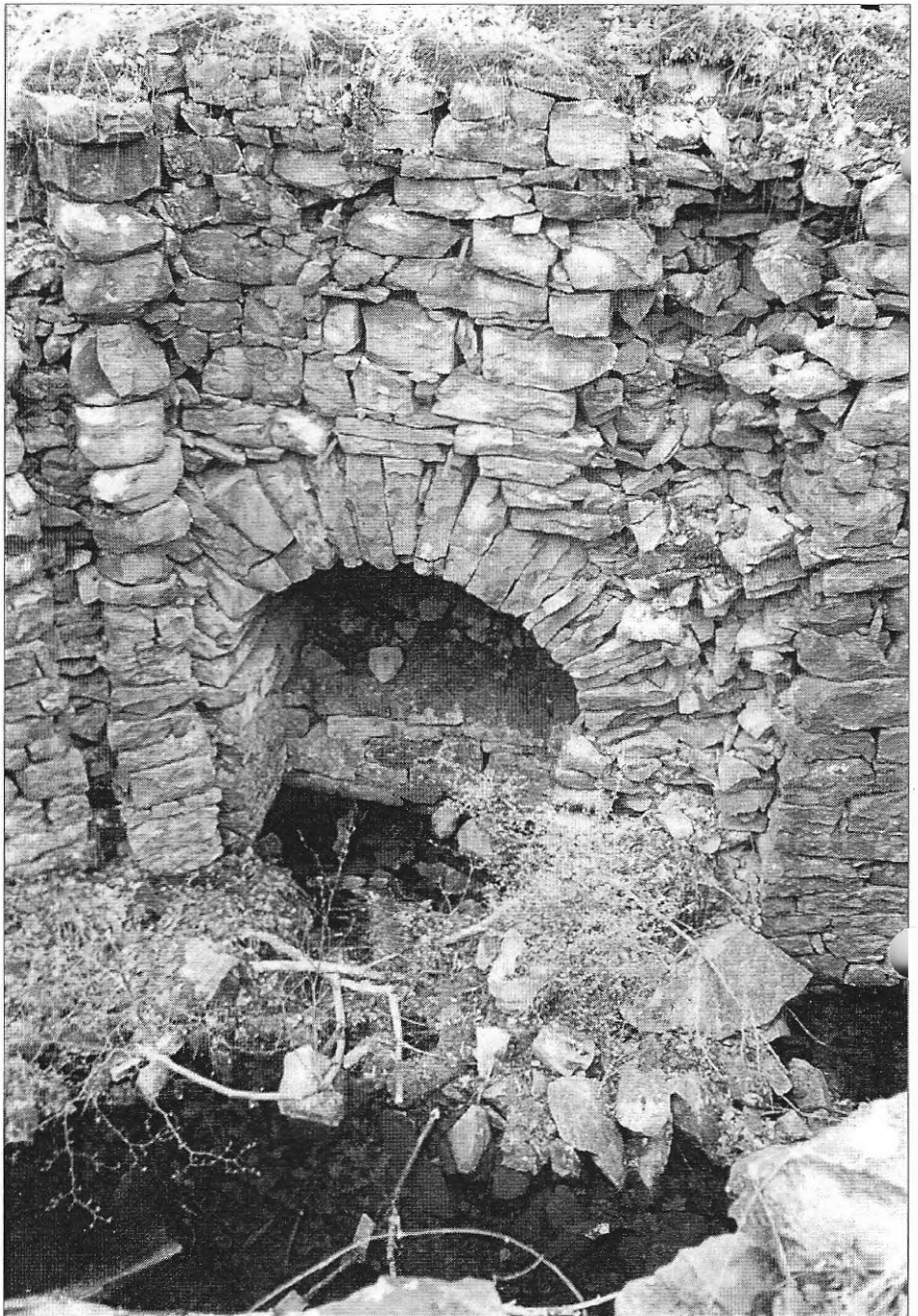
Close-up of one of the tunnels used to drain water from the bottom of the lock on the Upper Lehigh Canal. Use of such tunnels enabled a lock to be emptied in three minutes. Note the use of crude, rubble stone held together without cement. Construction dates to the 1830s.
