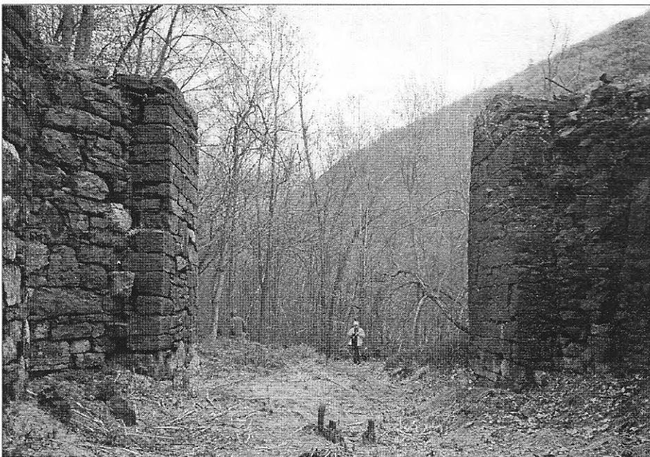
View of Lock 27, the second tallest on the upper division with a lift of almost thirty feet.
