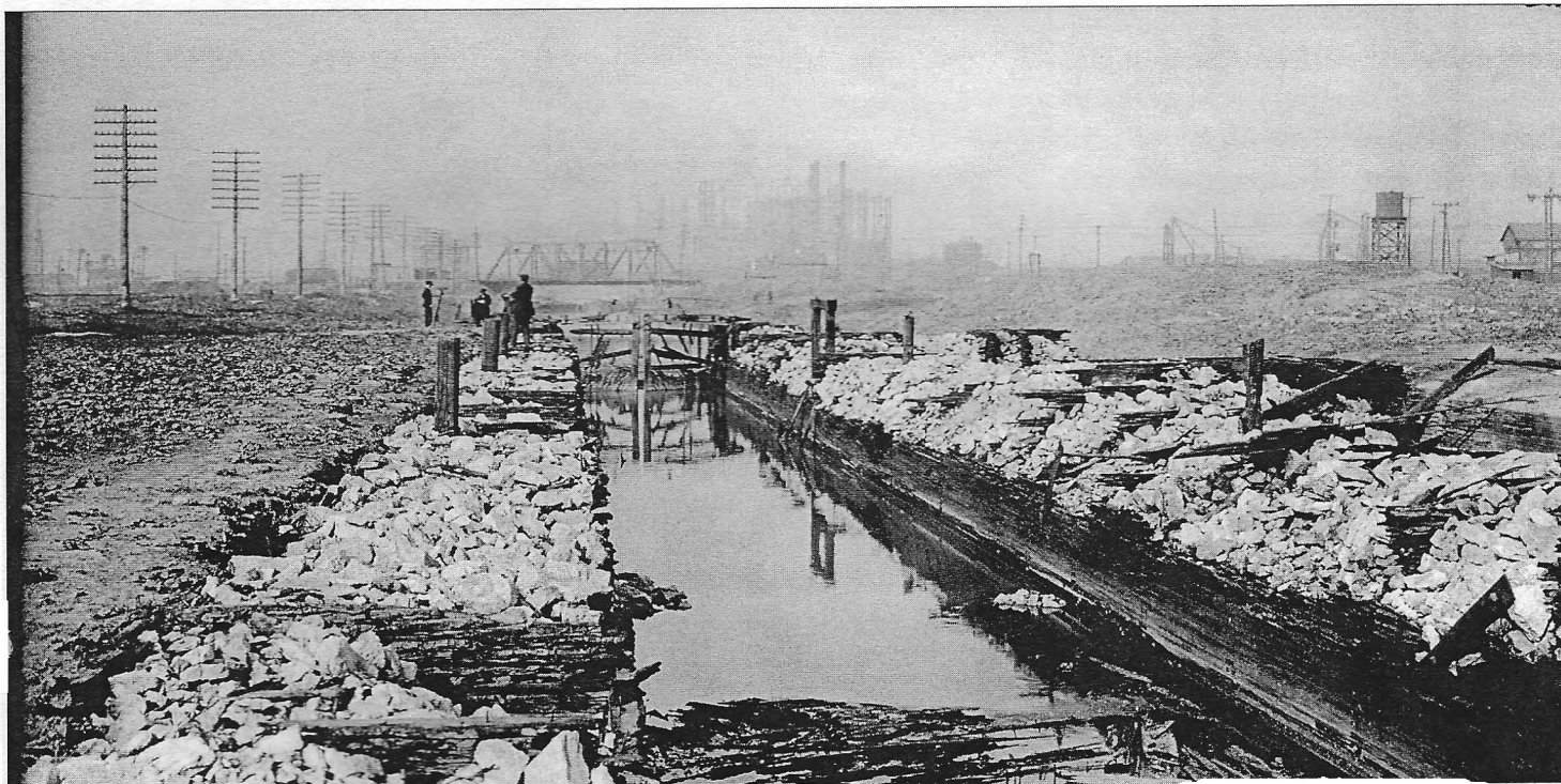
Bridgeport Lock looking north showing wood cribs 5/2/14
