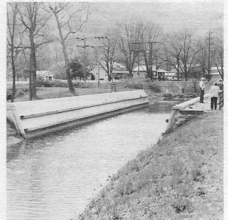
The restored canal channel, running across the Allegheny Creek Aqueduct at Gibraltar.
