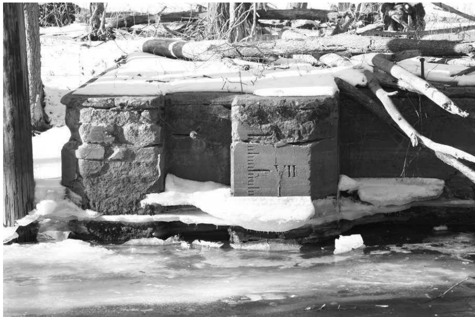
Hennepin Canal Lock 1, stop plank groove to west of upper gate showing depth gauge. Photo taken on 2/13/04 by Russ Price.
