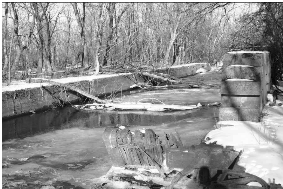
Hennepin Canal Lock 1, view across lock from upper towpath gate to lower berm gate recess with upper gate remains. Several piles of blocks on right hand wall are unexplained. Photo taken on 2/13/04 by Russ Price.
