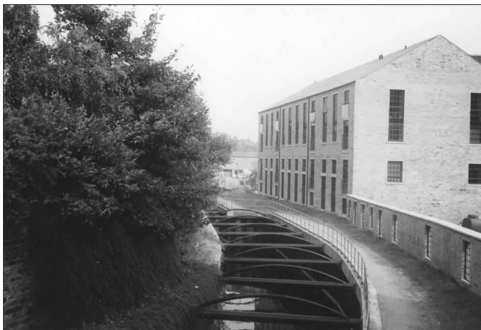
A portion of the Huddersfield Narrow Canal, in Huddersfield, required these support beams to prevent the stone retaining walls from caving in. Photo by Bruce Russell
