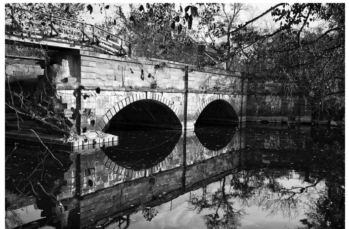
The first and second arches of the Seneca Aqueduct. The third arch was washed out by Hurricane Agnes in 1972. Photograph by Steve Dean
