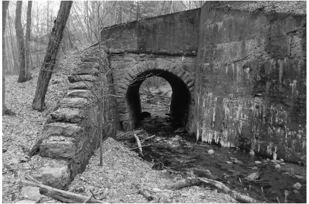
Above – Solomon Creek culvert under new Plane 2. Stonework likely dates to 1867-68 when the planes were rebuilt and new Plane 2 replaced old Plane 2, which is left of the picture. Concrete was probably added in 1908-09 when the planes were again rebuilt and concrete was used extensively.
