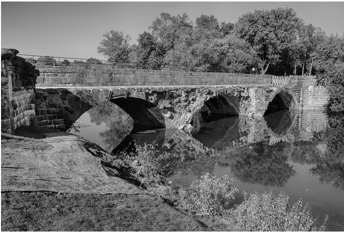
The Conococheague Aqueduct as it appears before the restoration project. Photo by Steve Dean
