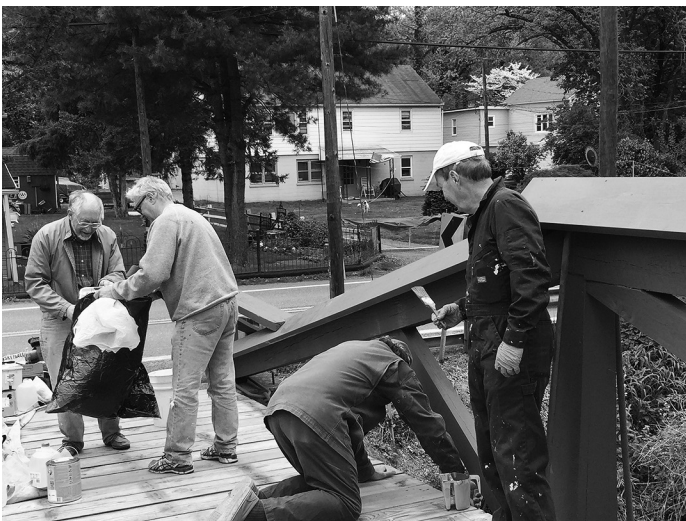
Friends of the Delaware Canal volunteers give Woody's Camelback Bridge its final coat of barn red stain. Photo courtesy of FODC
