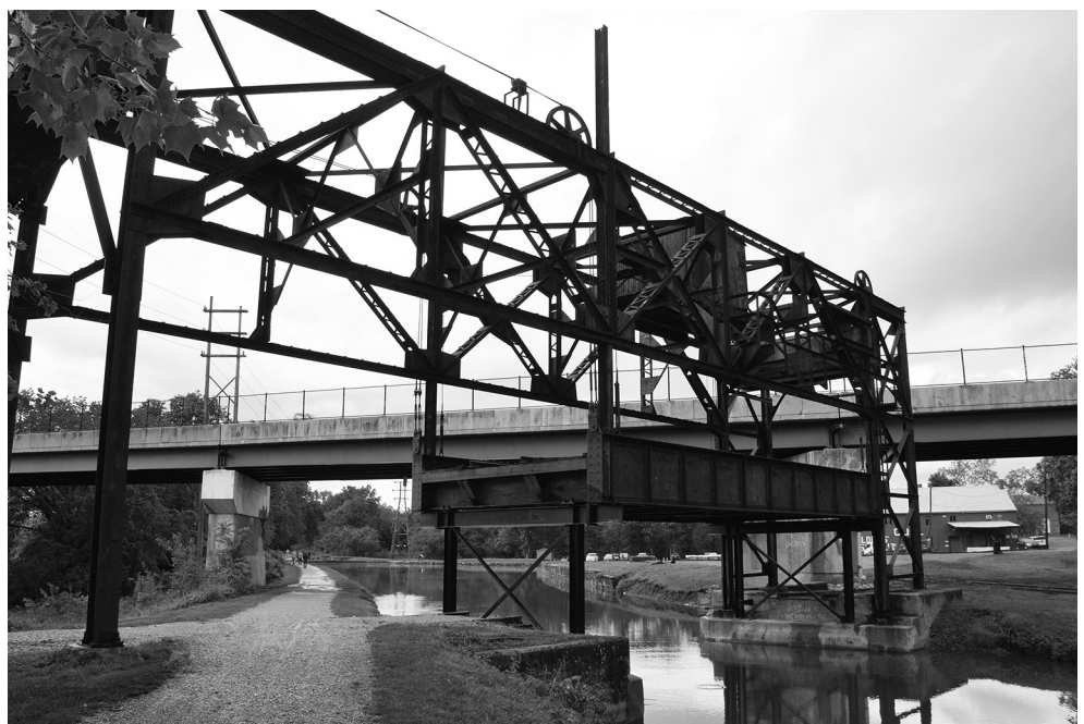
Western Maryland Railway lift bridge over C&O Canal. Photo by Gordon Perry
