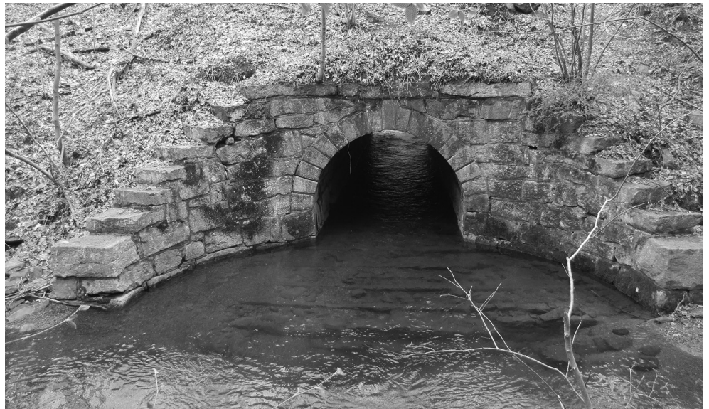
Below – Another culvert, this one on Plane 3, still on Solomon Creek. The stream here zig-zags as it goes through the culvert, essentially following the plane on one side, then along the opposite side. Photos by Doug Logan.
