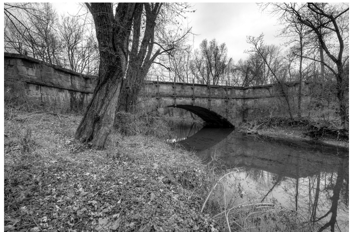
Evitts Creek (mile 180.66) – This is the uppermost aqueduct on the canal, and is four miles below Cumberland. It is stable, with support structures in place.
