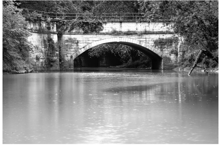
Fifteen Mile Creek (mile 140.90) – This aqueduct is easily accessed and viewed in Little Orleans, Md. It is in excellent condition, with both the towpath and berm walls intact.
