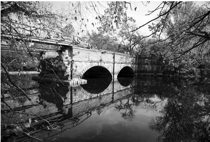
Seneca Creek (mile 22.82) – This three-arch aqueduct is made from red Seneca stone. A local flood in 1971 washed out the upstream arch. It is combined with a lift lock.
