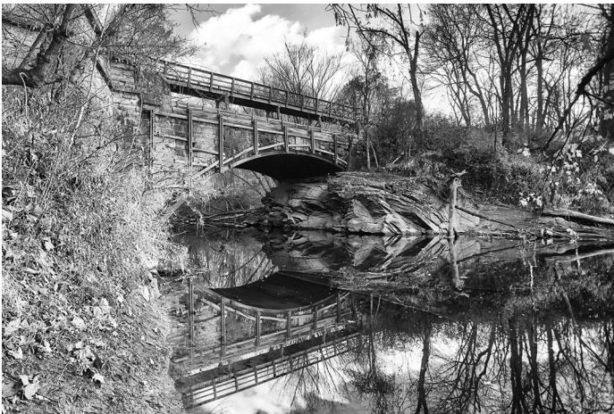
Tonoloway Creek (mile 122.96) – Located in the canal town of Hancock, this aqueduct features an irregular arch that rests on a rocky ledge on the downstream side.
