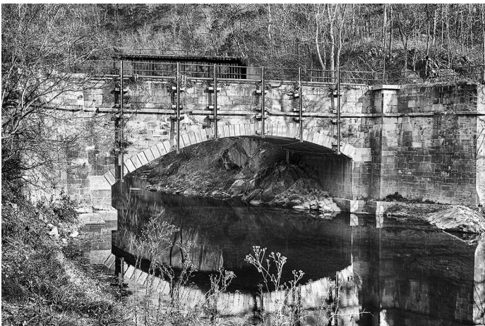
Sideling Creek (mile 136.56) – This aqueduct is located in a quiet area at the foot of Sideling Hill. It features a 60-foot asymmetrical arch.
