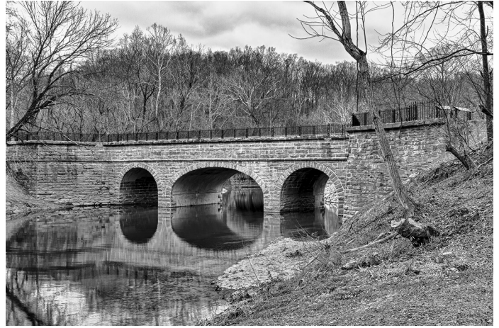
Catoctin Creek (mile 51.53) – Two of this aqueduct's three arches collapsed in 1973. A restoration project was completed in 2011 and used many of the original stones
