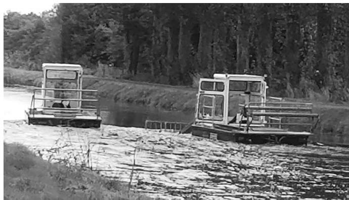
Vegetation clearing at Boland's Lock, lock #26, on the Grand Canal. The first boat cuts the vegetation in the canal with a blade that looks like a giant hedge trimmer. The second boat rakes up the cut vegetation. – Photo by Rod Mackler
