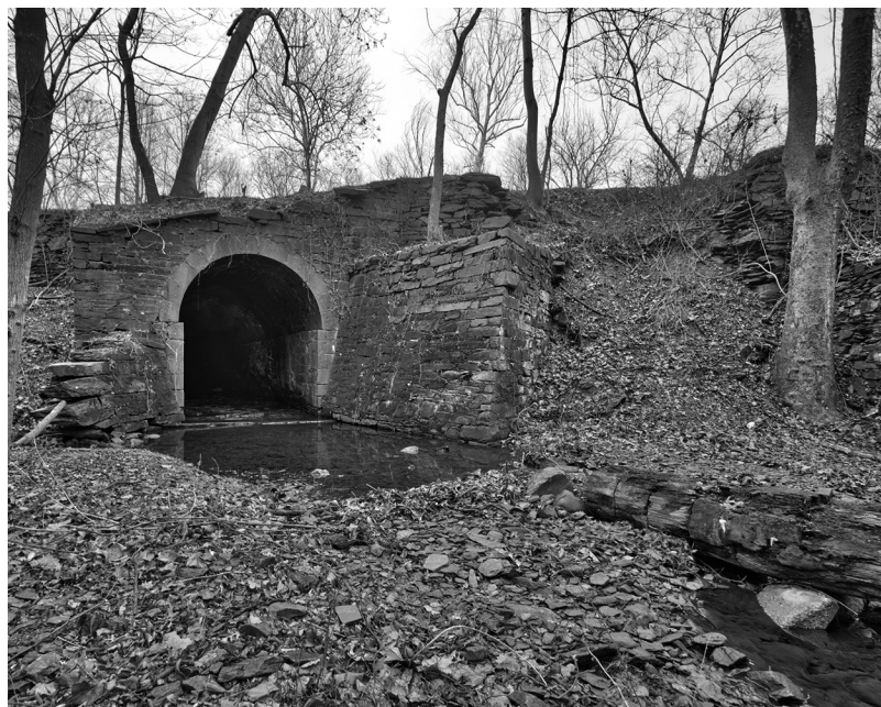
Rock Run Culvert (Mile 8.93). Note the retaining wall failure on the right – Photo by Steve Dean
