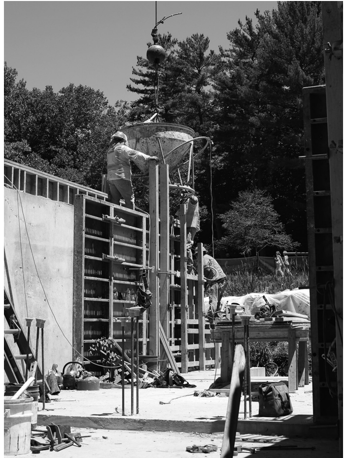
Construction workers pour concrete to form the walls of the Lock 20 waste weir replacement – Photo by Stephanie Spencer
