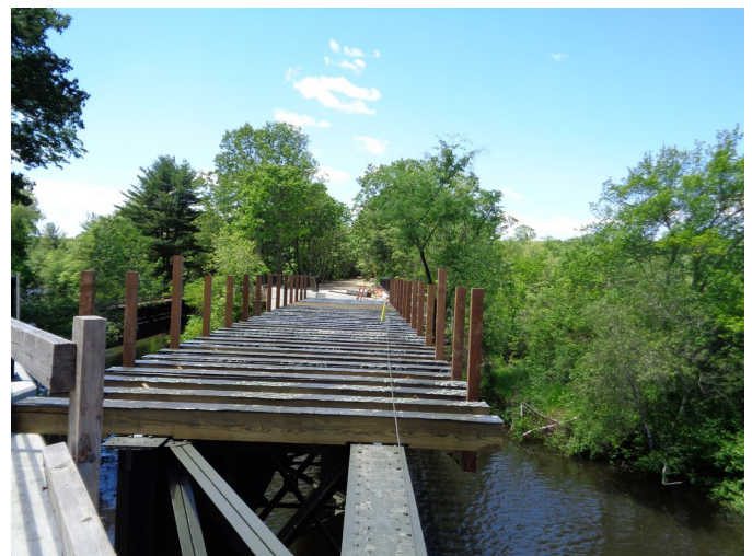
The shorter Factory Pond Bridge looking west on 6/15/14 showing the deck and railings under construction
