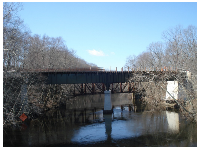
The bikeway Blackstone River Bridge in Blackstone with most of the decking installed and some of the handrails completed. on 4/9/14
