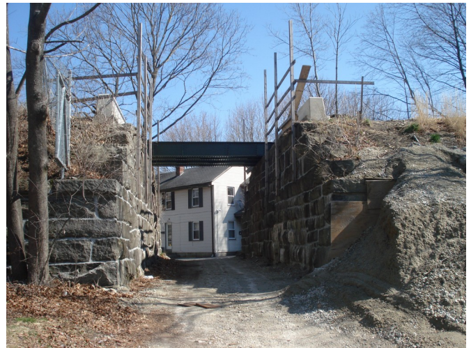
As viewed on April 9, 2014, the Kane Court bikeway bridge in Blackstone has been returned to its site after being rehabbed and repainted elsewhere and now awaits decking and handrails.
