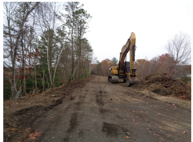
View east along SNETT at Adams St. parking lot, just east of Rte. 146A on 11/2/14
