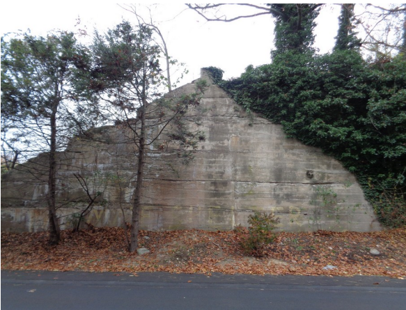
The north abutment for the “Titanic Railroad” Bridge at Castle Hill Way, Bellingham
