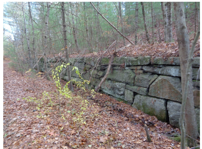
View eastward on the SNETT just west of Prospect St., Franklin showing the high masonry wall on the south side.
