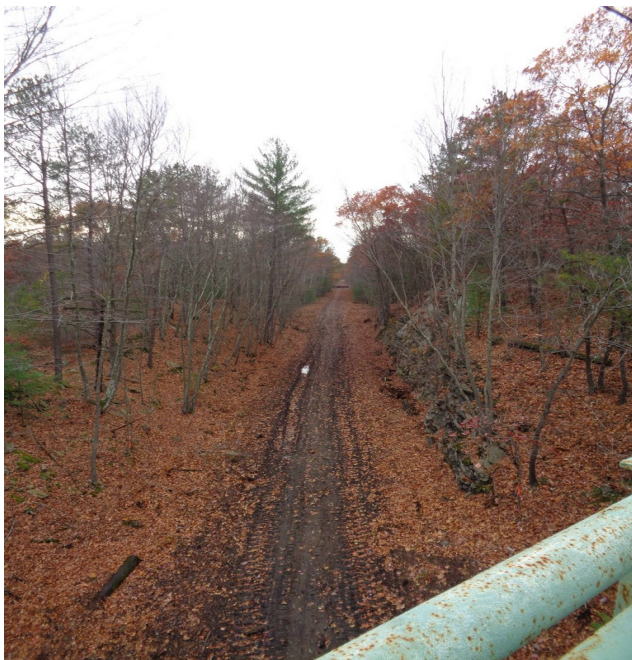
View of cleared SNETT looking west from Rte. 126 on 11/2/14 with Triad Bridge in the background.
