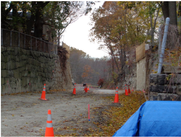
Telephoto view from Old Mendon Rd. to Factory Pond bridge in Blackstone on 11/2/14
