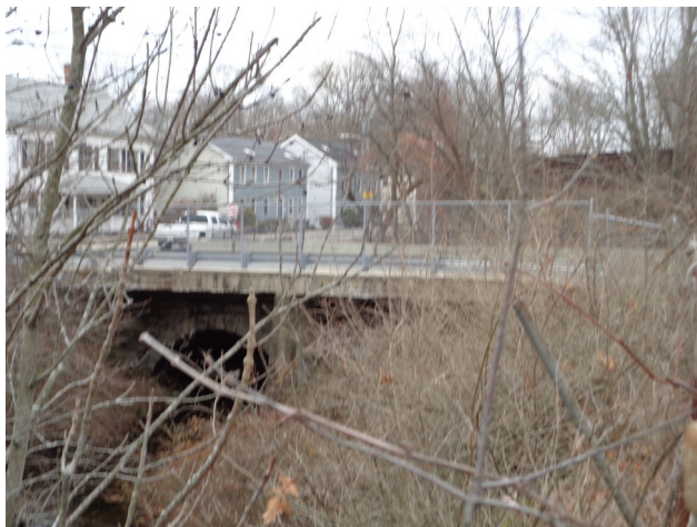
North view of the St. Paul St. Bridge in Blackstone 11/25/14. The left arch is visible under the concrete sidewalk, but the right arch is totally obscured.
