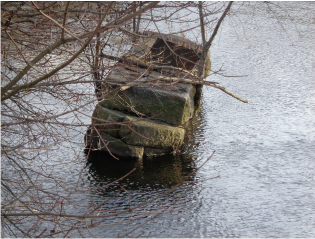
The damaged, in river pier from the original bridge. The undermining of this pier caused the removal of the bridge and closing of the rail line to Franklin.
