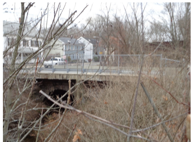
The St. Paul St. bridge viewed from the north with undergrowth blocking the view of the right arch. Also shown is the later concrete sidewalk.
