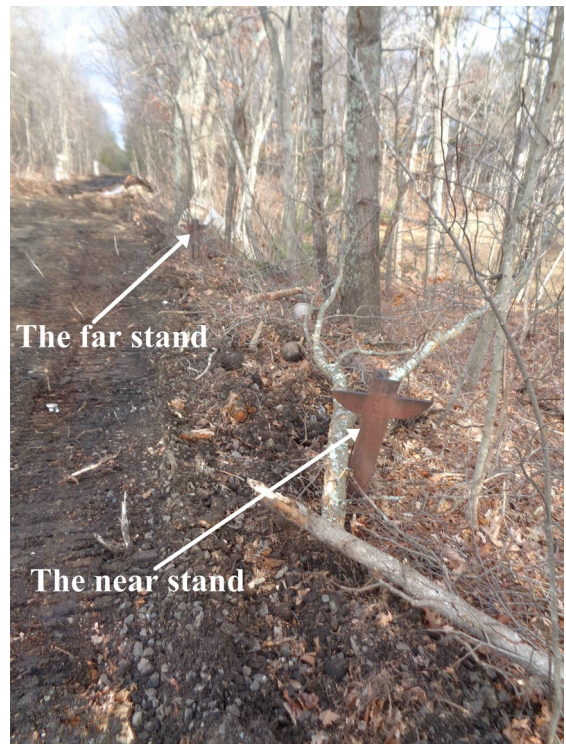
The set of spare rail supports just east of Center St., Bellingham
