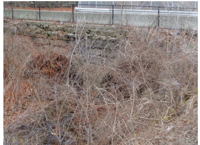
The 1851 St. Paul St. bridge viewed from the south showing the overgrowth in the canal.
