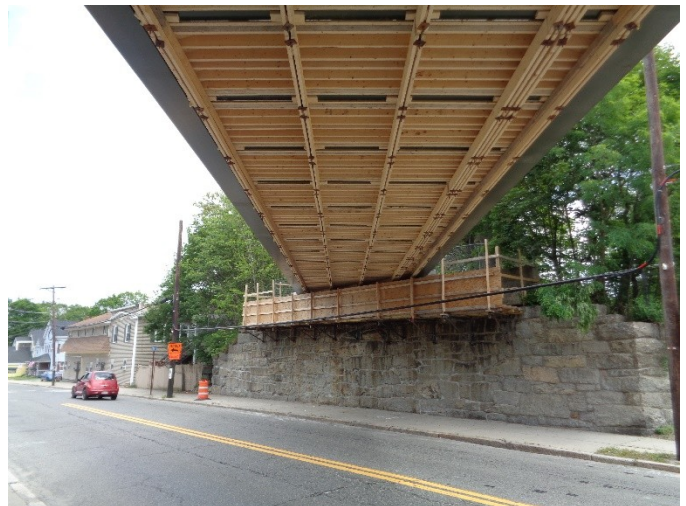
Under side of the new Main St. Bridge, Blackstone ready for deck pour 6/20/15
