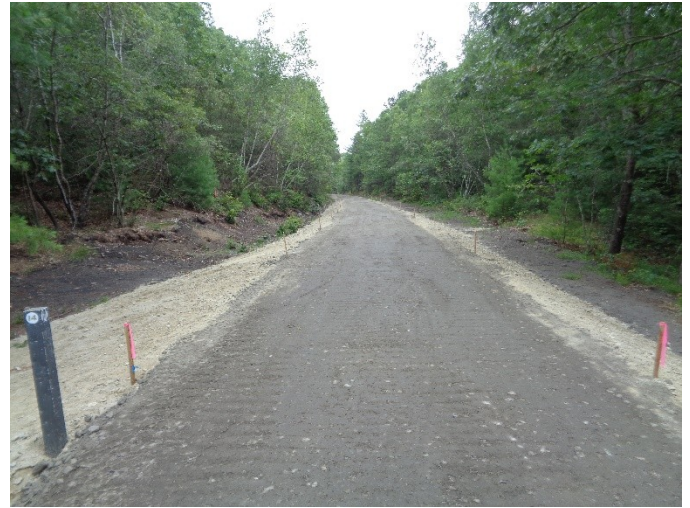
View looking eastward at the side trail to Millville Lock on 7/18/15 showing the newly installed base material
