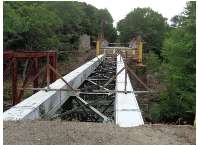
View eastward across the SNETT Bridge at the Triad Bridges on 7/18/15 showing the new paint work. On the left edge is the P&W Bridge (rusted steel). Between that bridge and the yellow steel of the SNETT Bridge is a concrete pier for the never completed Southern New England Railroad Bridge which would have crossed over the SNETT Bridge. Looking through the middle of the yellow SNETT Bridge, the Route 122 highway bridge is visible in the distance. Shortly, a wooden deck will be installed on top of the steel.
