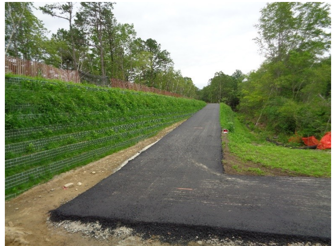
The newly paved ramp from the Adams Street parking lot, Uxbridge up to the SNETT looking east on 7/18/15. Note the stabilized embankment on the left.
