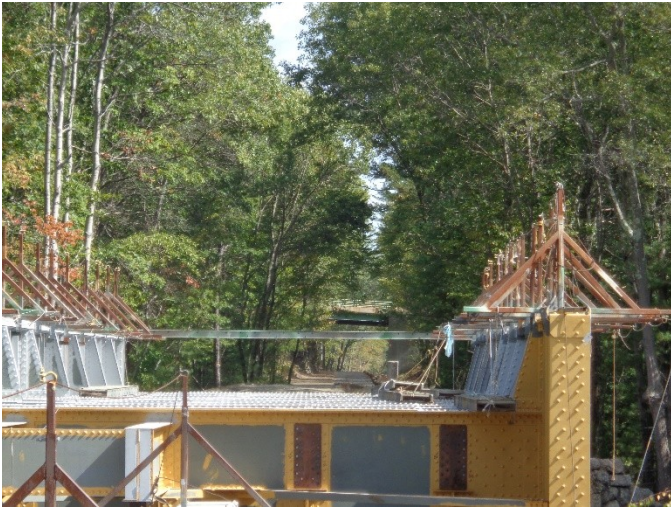
Telephoto view east across the Triad Bridge to the Rte. 122 Bridge on 9/26/15. Paved bikeway can be seen on the far side.
