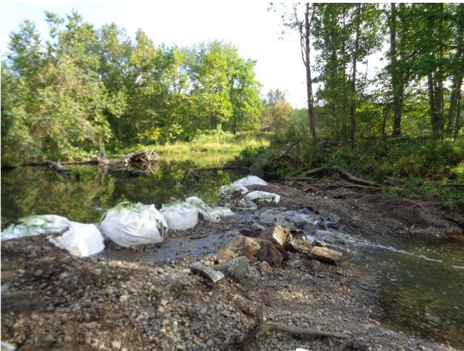
The dam just south of the breach on 9/19/15
