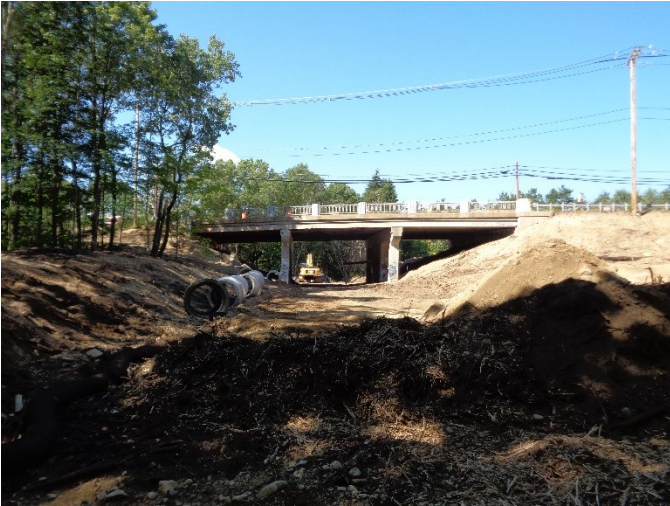
View of the work underway to replace the Rte. 126 Bridge in Bellingham looking west on 8/8/15.
