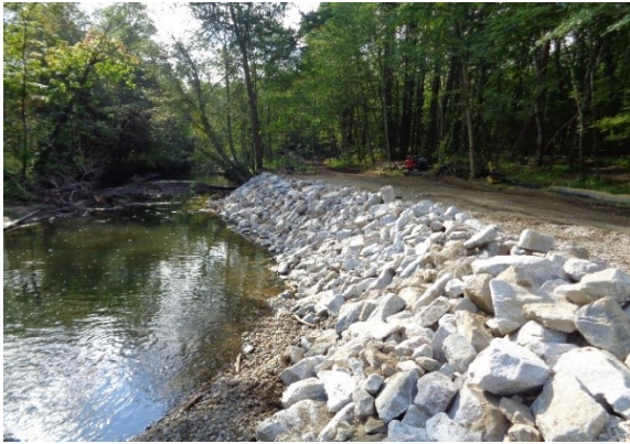
New riprapping on the west bank of the canal, looking south, at the north breach on 9/19/15
