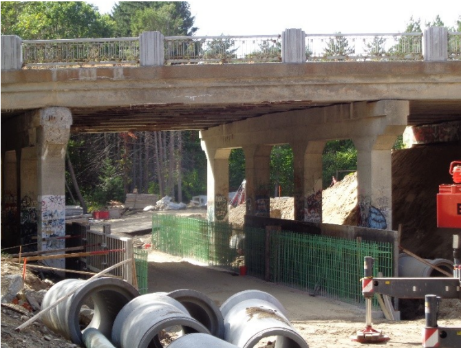
Rte. 126 tunnel work on 9/26/15. The tunnel floor is cast and rebar and form work is in process on the side walls.
