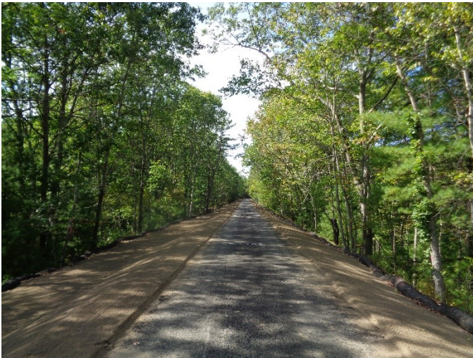
View west along the bikeway west of the Triad Bridge on 9/26/15 showing pavement with new top soil on each side
