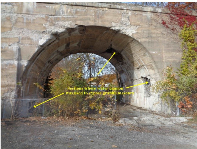
Eastern arch of the seven arch viaduct showing areas where masonry was exposed by water cannon.
