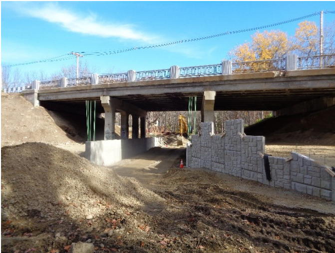
View of the work underway to replace the Rte. 126 Bridge in Bellingham looking east on 10/31/15.
