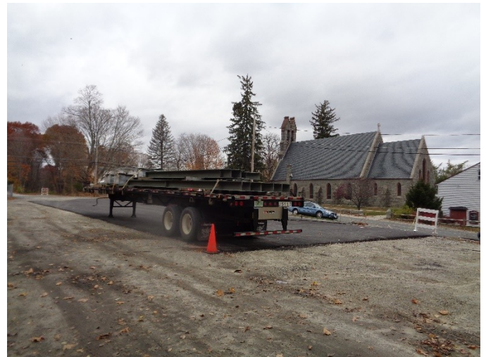
Steel beams & pedestals at Central St., Millville on 11/1/15. These are to be installed on the Triad Bridge.
