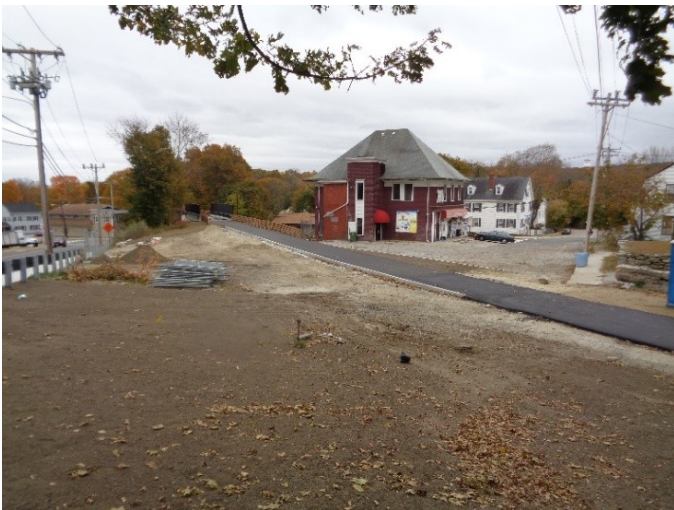
View of the Old Mendon St. area on 10/2/15 looking towards the old firehouse and the Main St. Bridge. All fencing is now gone. Fencing remains across the end of the Main St. Bridge and at the entrance to the tunnel cut.
