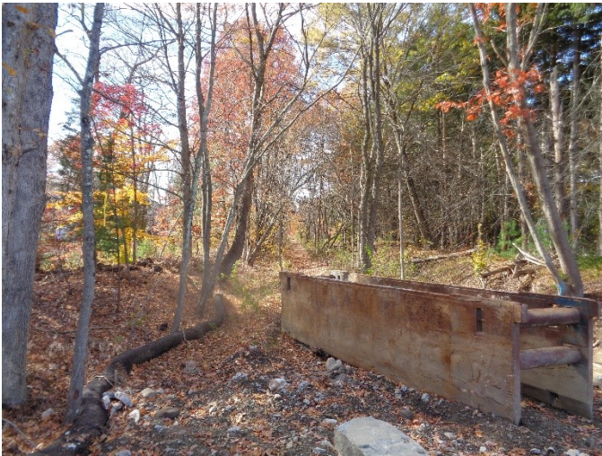
View of the SNETT looking west from the present Rte. 126 tunnel construction on 10/31/15.
