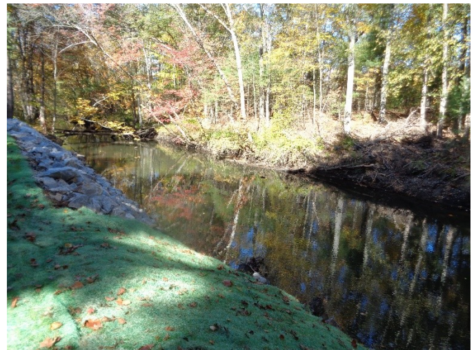
Finished canal repair work where the downed trees that used to strain debris south of Church St., Northbridge once were.
