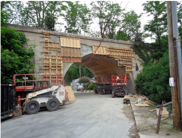
The south face of the middle arch of the Blackstone Viaduct on 7/10/16
