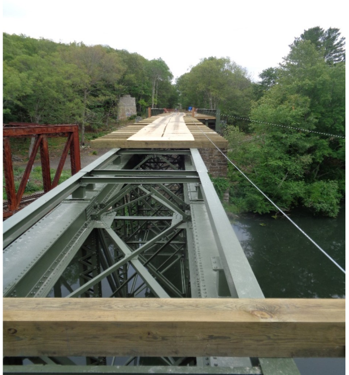
View east across the Triad Bridge on 7/10/16 showing new decking being installed
