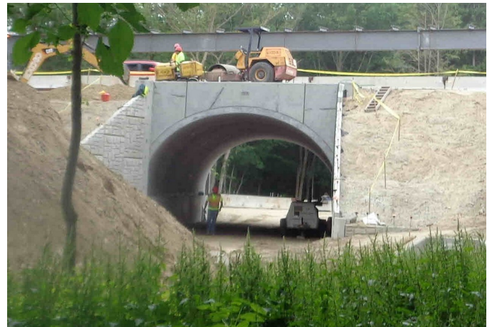
The new tunnel under Rte. 126 in Bellingham after removal of the old bridge. The gray steel beam supported a water line during the change and has since been removed.
