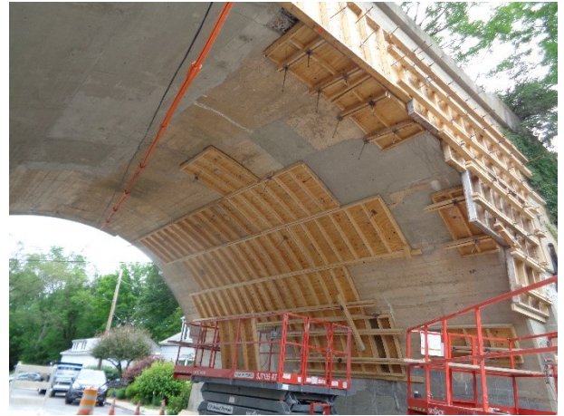
Formwork and new concrete in the Blackstone Viaduct SNETT Rte. 126 Tunnel Progress
