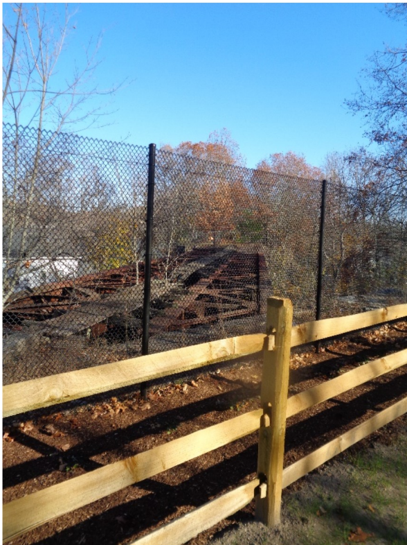
View eastward across the Norfolk County Railroad Bridge over the Blackstone Canal and Canal Street in Blackstone on 11/13/16. In the future, the route will cross this bridge and the Blackstone Viaduct just beyond to connect up with the Greenway in Rhode Island.
