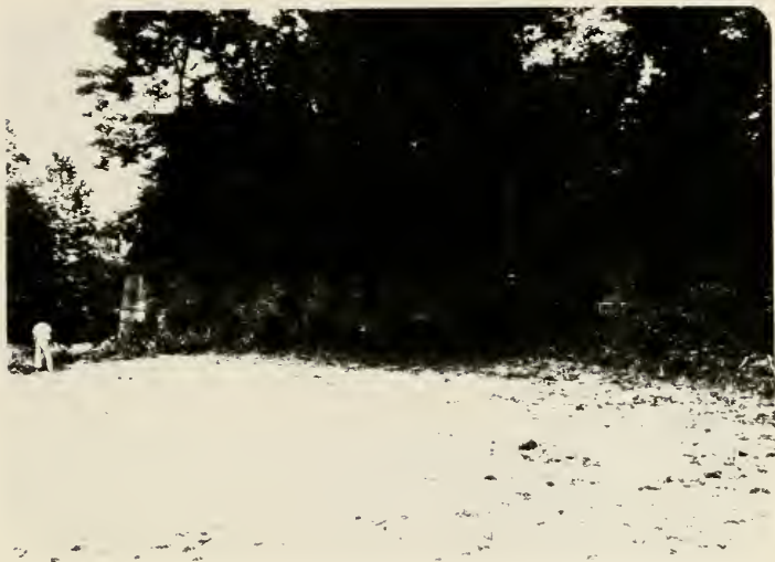
Plate 49. South wall of the eastern abutment of Hay Creek Aqueduct, photographed in 1989.
