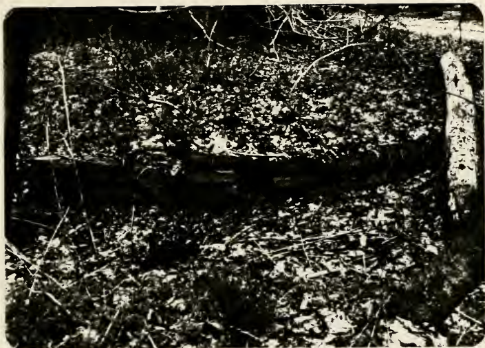
Plate 87. Small stone pier on north bank of the canal for Grubb's Farm Bridge.
