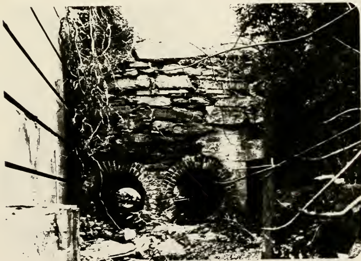
Plate 46. Dual sluice pipes in the basin below Lock 51 which appear to have fed water to the Birdsboro shop.
