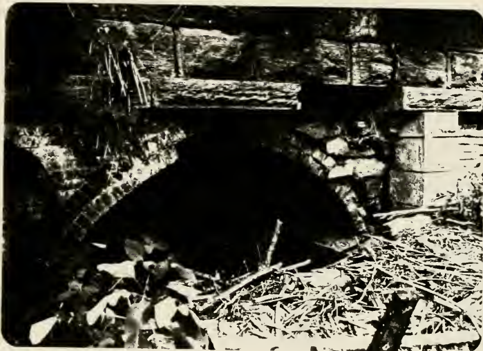
Plate 27. Damaged arch in the south wall of Seidel's Aqueduct.
