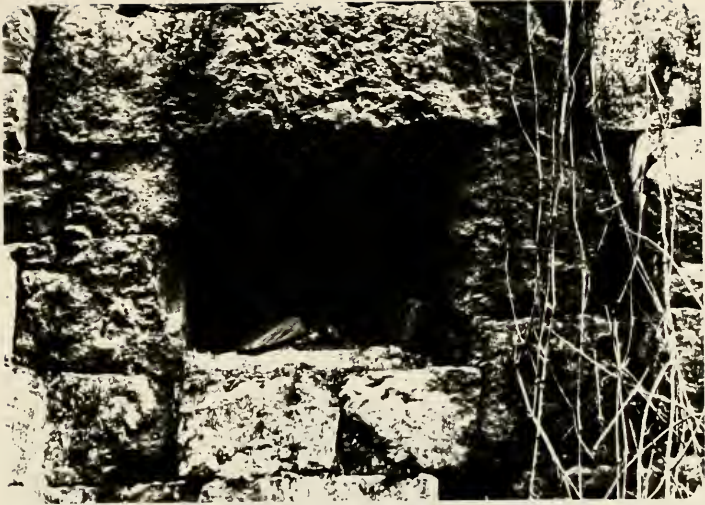
Plate 76. Detail showing one of the drainage culverts built into the lower chamber at Laurel Hill Locks.
