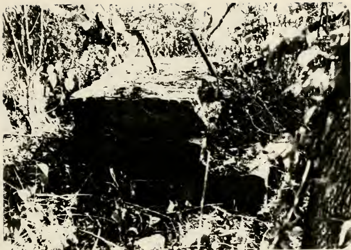
Plate 66. Ruin of a stone pier which supported the timber work at Kirlin's Aqueduct.
