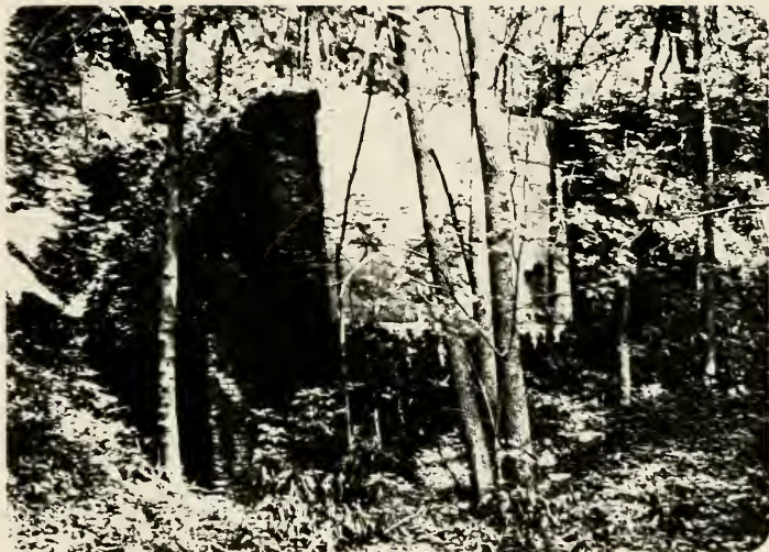
Plate 15. Dam abutment on the north side of the Schuylkill River near the site of the Klapperthal hydro-electric plant.
