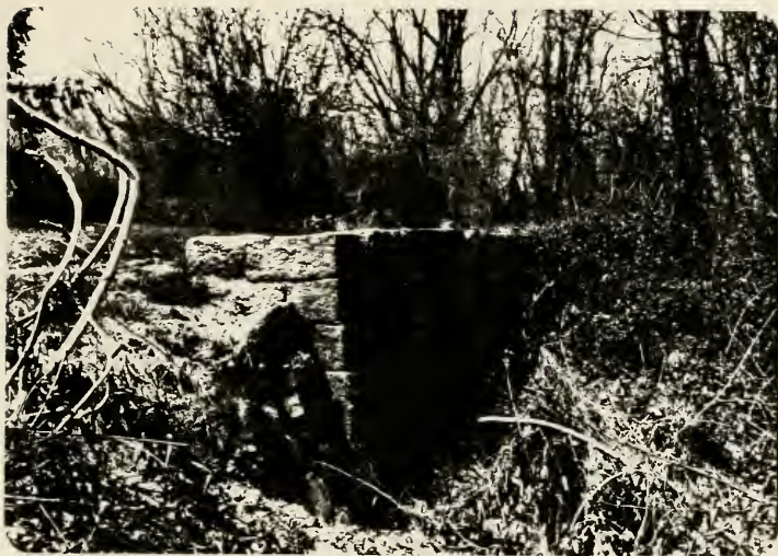
Plate 93. Possible fragment of the western abutment of the tow path bridge over Lock 55 at Frick's Locks.
