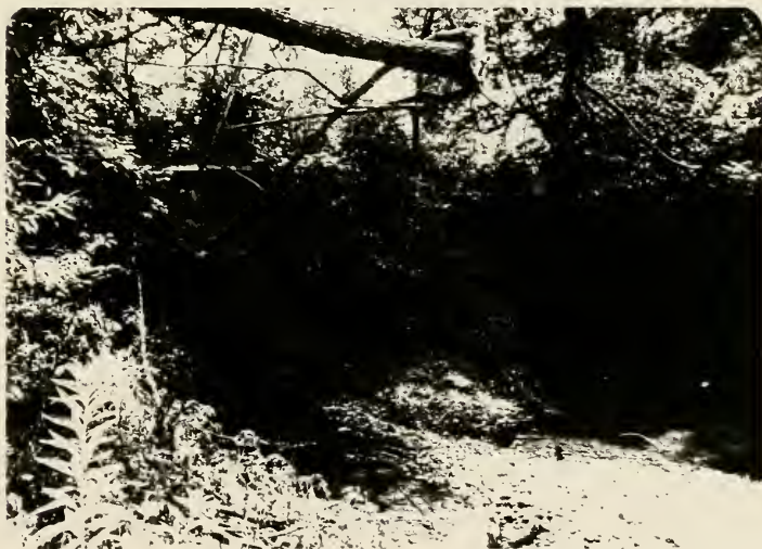
Plate 25. Seidel's Aqueduct viewed from the north; note the waste weir built into the wall of the structure.
