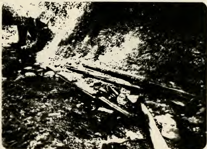
Plate 32. Remains of timber work aqueduct built to replace Haw's Double Culvert in 1874.
