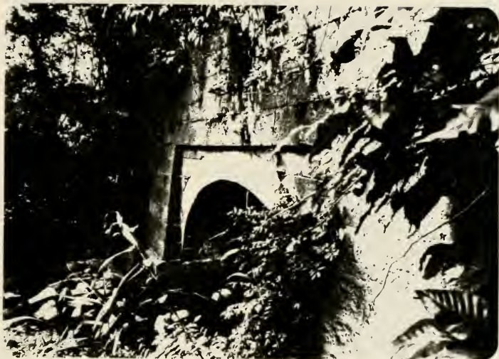
Plate 29. Detail of south wall of Haw's Double Culvert showing center pier and arches.
