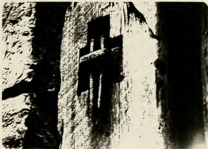
Plate 81. Beam held by iron anchor assembly outside the lower gate of Lock 53 at Laurel Hill.
