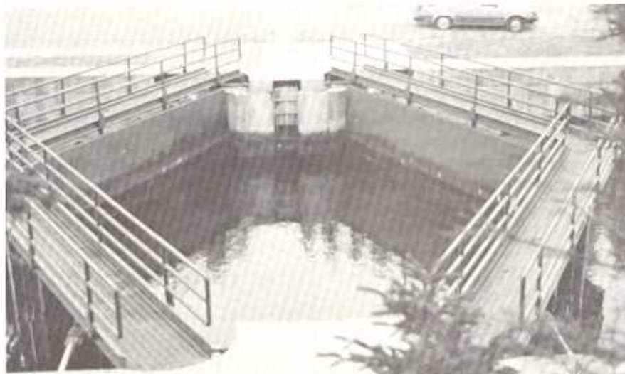
ST. PETERS CANAL, 1987. A PAIR OF MITRE GATES AT THE EAST END OF THE LOCK. Photo by Colin Duquemin
